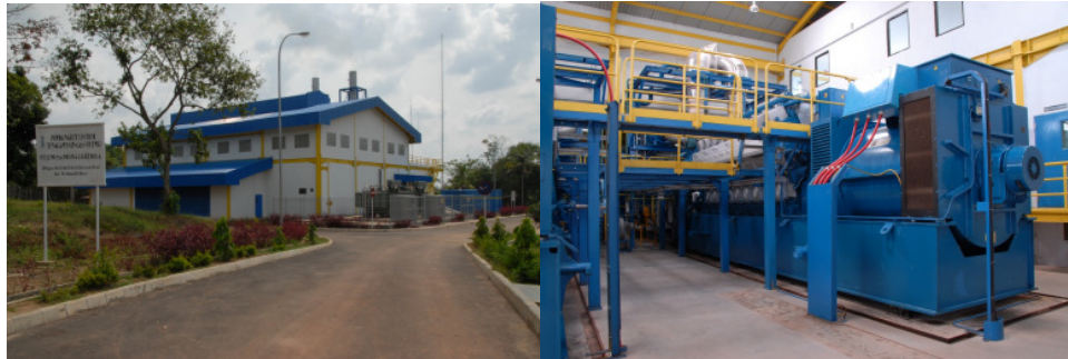
IPP Musi II 3 x 4.7 MW Gas Turbine Power Plant
